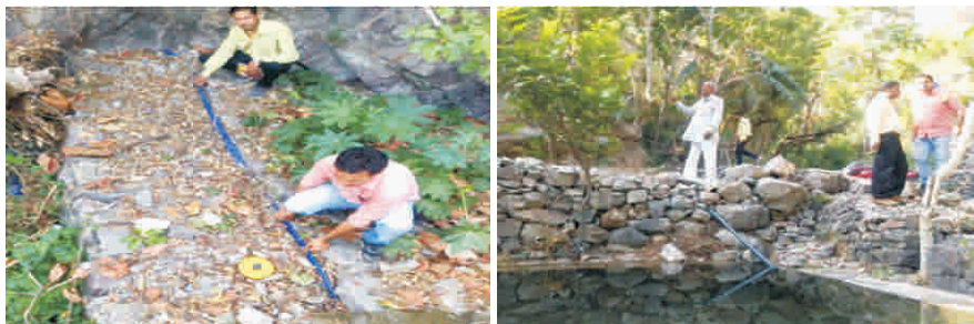
Fig.23 : Embedded checkdams: Dharkot-1 (L) and Dharkot-2 (R) constructed at Dharkot, Dehra Dun
