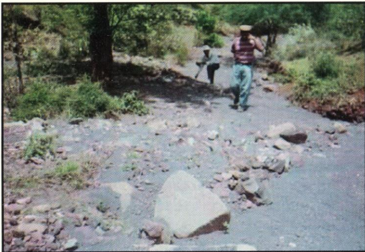
Plate 3. A steep nala which has stabilized after construction of a series of gabions
