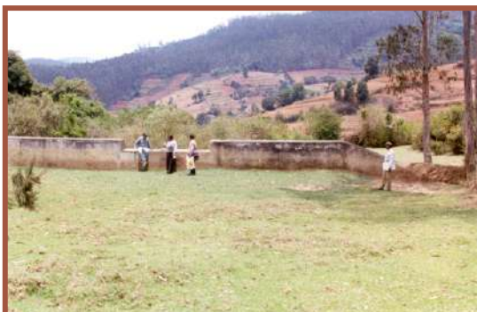
Silted up check dam before project intervention at Kavakadu
