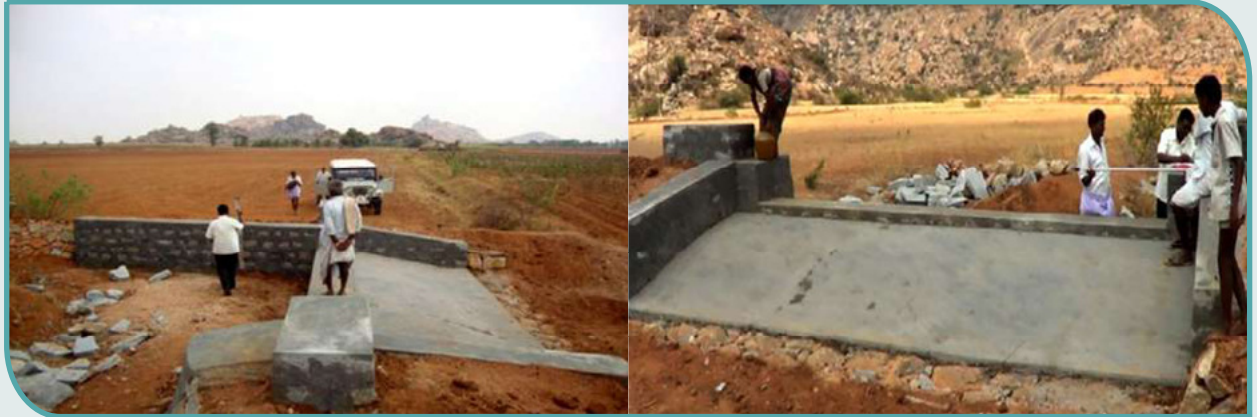
Fig. 5.8. Check dam cum drop weir with retention wall and embankment
