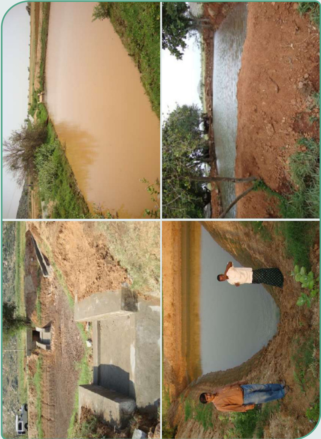
Fig. 5.12. Percolation tank and fish pond cum water storing structure in nala course and arable lands
