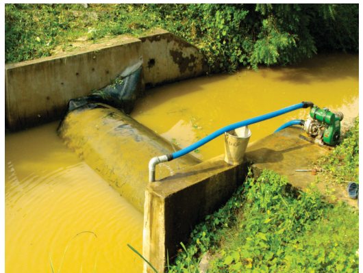
Flexi check dam
