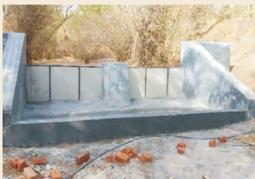
Cost Effective Plastic Check Dams for Water Harvesting in Rainfed Regions
