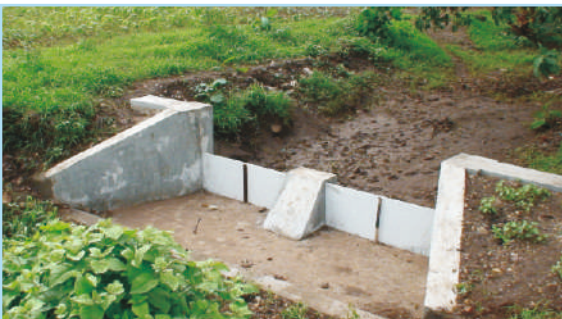
Plastic head wall embedded composite check dams for reducing the cost of construction and easy construction in remote location in ravine
