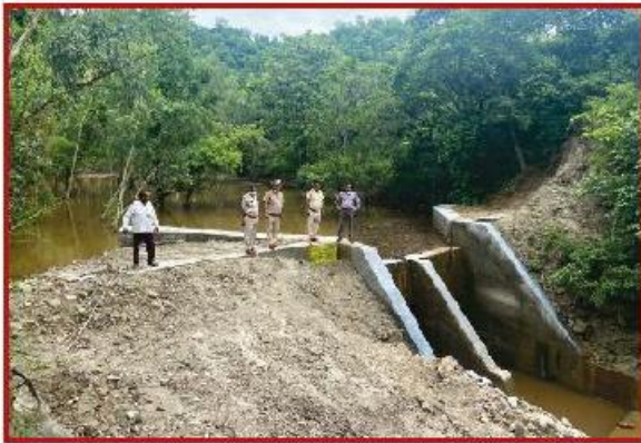
Photo 4.5: Straight drop spillway with Earthen embankment at Ranjeetpur block, Yamuna Nagar, Haryana
