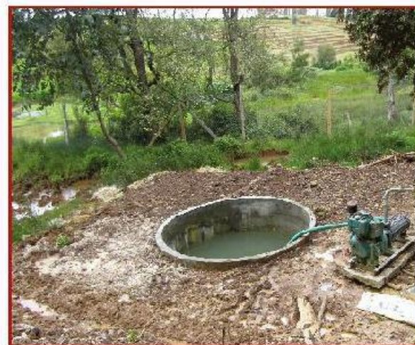
Photo 4.37: Collection well for sub surface water harvesting, Tamil Nadu
