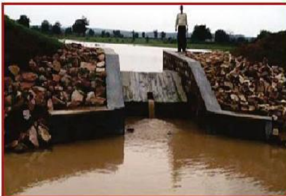
Photo 4.9: Straight drop spillway, Uttar Pradesh
