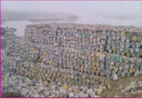
Katta-Crate Technology: A Cost Effective Measure for Rehabilitation of Torrents and Minespoil Areas
