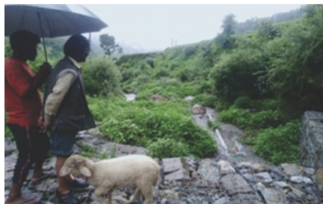
Farmers inspecting check dam in Satyon village after the extreme rainfall event during 26-27 th August, 2021
