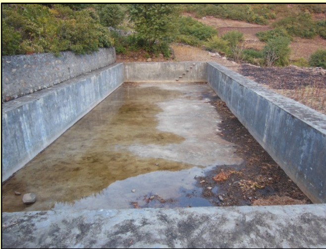
Non-Functional Water Storage Tank in Attal Village
